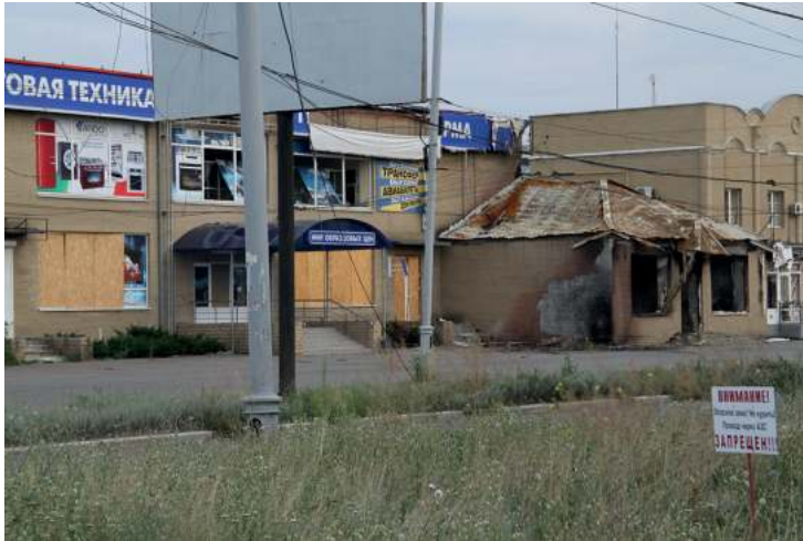
Damaged market “Slovyanskyi Bulvar” resulting from shelling on June 8, 2014. Photo credit: Kostiantyn Reutskyi, July 17, 2014
