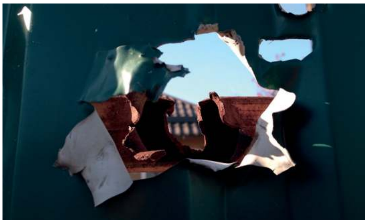
Fence damaged by debris in Cherevkivka. Photo credit: Mariia Biliakova, November 1, 2018
