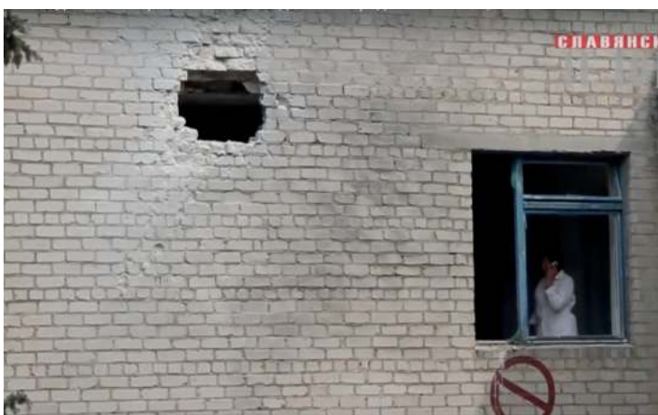
Damaged City Children's Hospital. Source: screenshot from the video on the YouTube channel "Delovoy Slovyansk", http://bit.ly/2jUaXXQ
