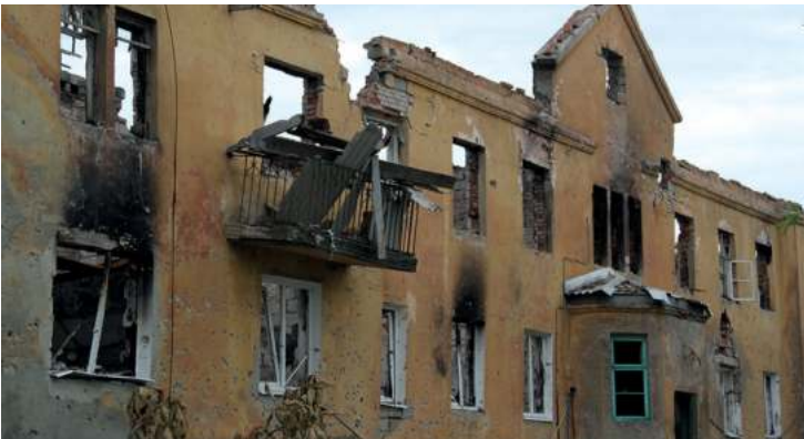
The destroyed building of the Psychiatric Hospital, Semenivka. Photo credit: Kostiantyn Reutskyi, July 19, 2014
