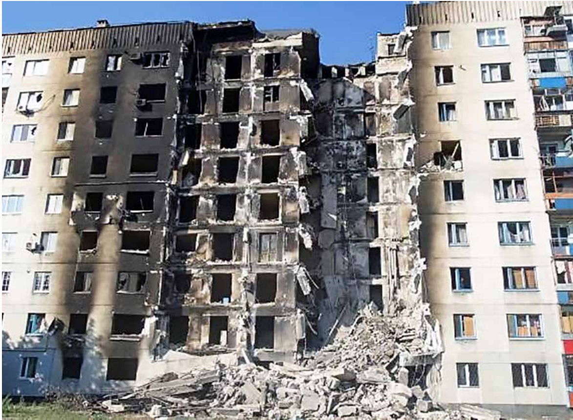
A destroyed building in Lysychansk — the former home of the respondent
