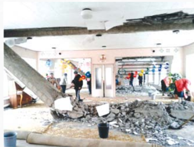
Ruined kindergarten “Nadiya” in Kirovsk
