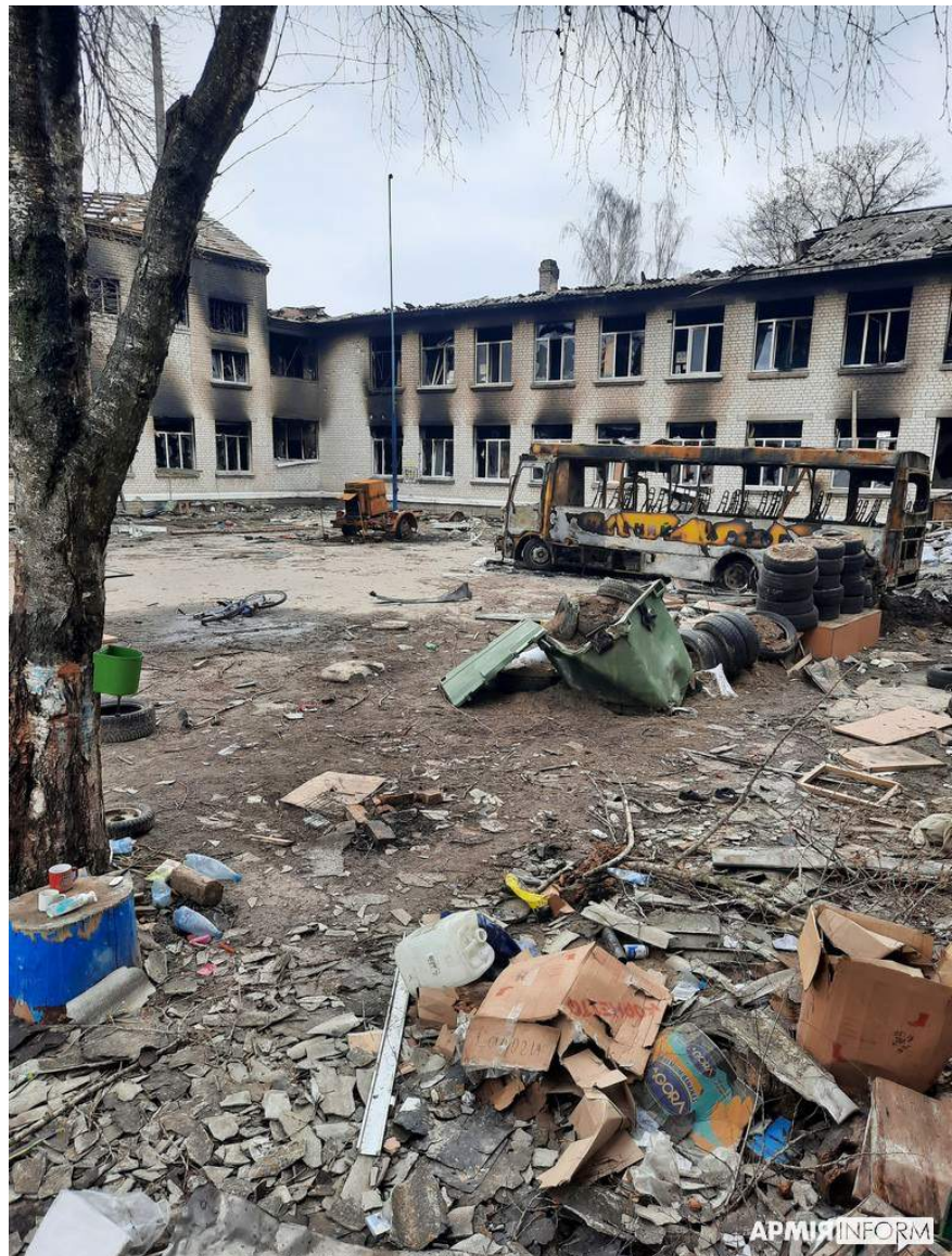
School in the village of Bohdanivka. Consequences of the armed aggression. Source: ArmiaINFORM
