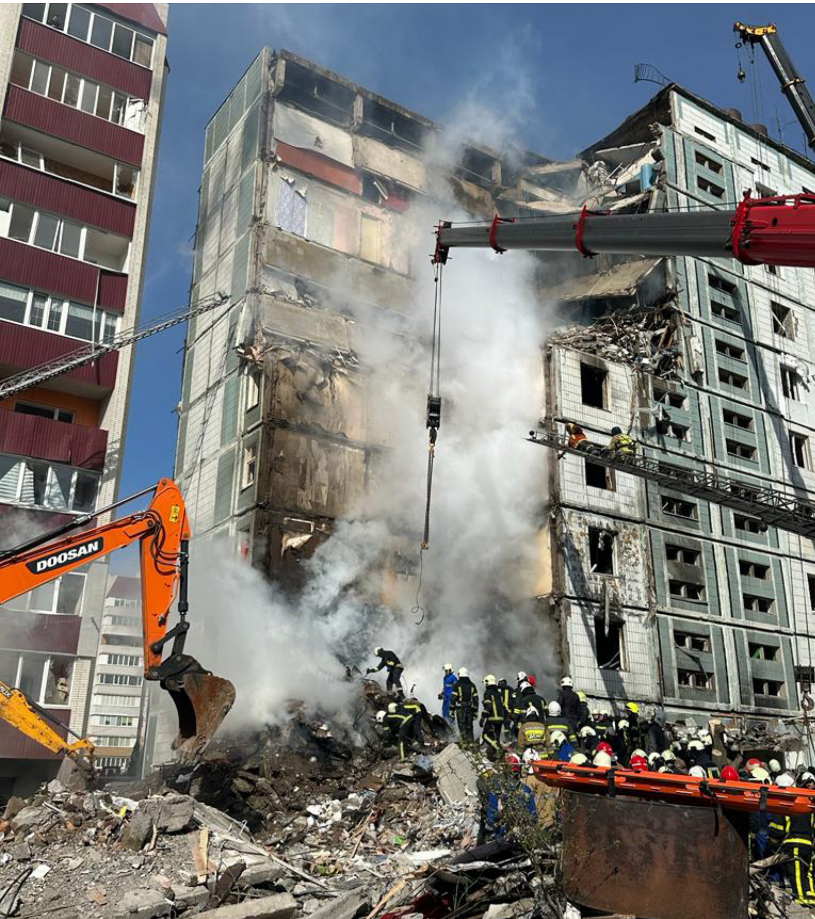
Rescuers clear the rubble of the nine-story residential building in the city of Uman after a Russian missile hit it. Photo source: State Emergency Service of Ukraine
